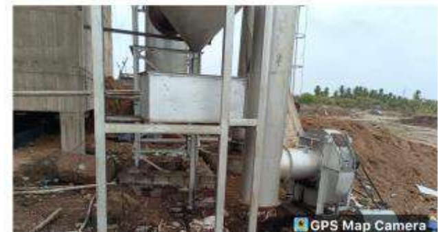
VENTURI WET SCRUBBER WITH ID FAN
